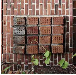
Perforaties in baksteen
